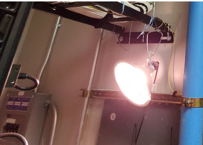
An example of non-compliant rack illumination.
