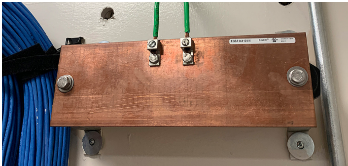
Due to undersized conductors and single-hole lugs, this Grounding infrastructure does not meet industry standards.
