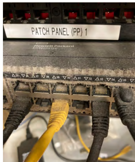
Dust and dirt are other environmental factors that can negatively affect equipment performance. These network switches and air vents are clogged with dust.
