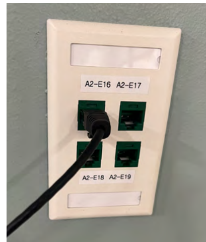
Whenever possible, data outlets shall be flush mounted. Labels shall be machine printed and not hand written.
