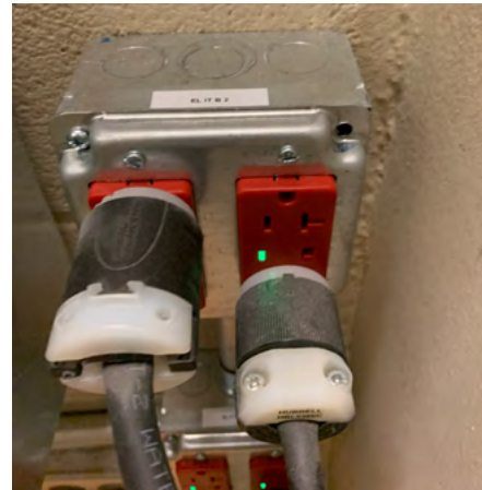
These emergency power outlets are correctly labeled and used in this TR.
