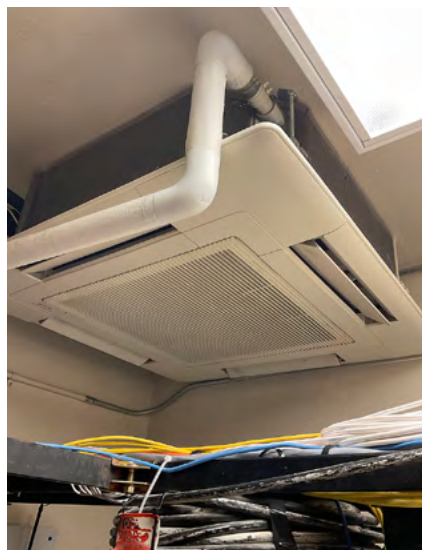
HVAC equipment must not be installed directly over a rack as it presents a water threat to the IT equipment.
