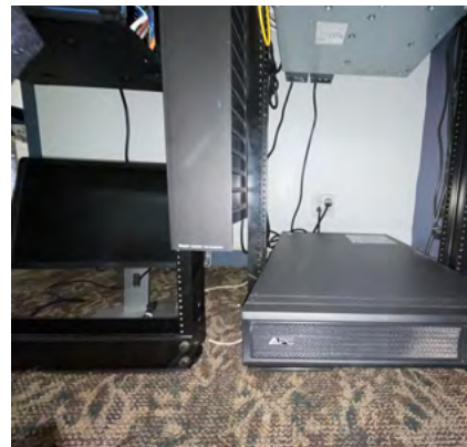
Carpeting is not a standards-compliant flooring type due to risk of ESD.
