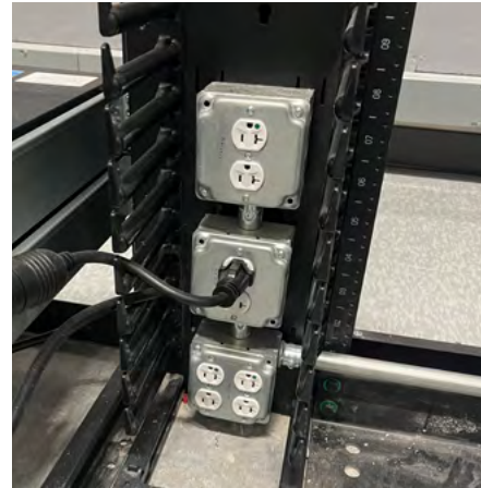
Electrical outlets should be mounted to all racks.
