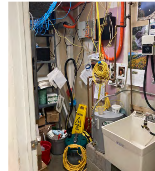
This TR is shared with a custodial closet with a utility sink that should not be in the space.
