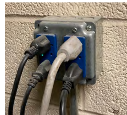
While a TR emergency power outlet is present and in use, it is not properly labeled.
