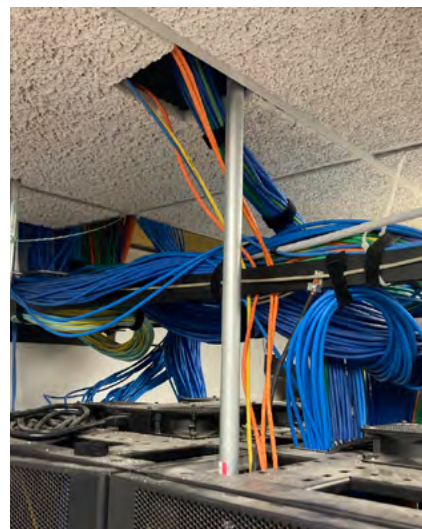
A non-compliant drop ceiling with tile cable cutouts in a TR.
