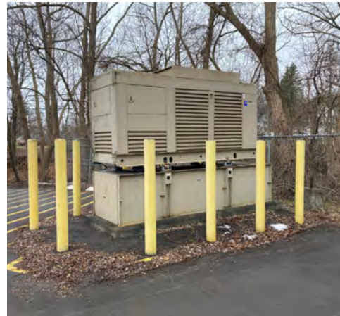
Building generators provide electrical power to connected outlets installed throughout the facility including in all TRs.
