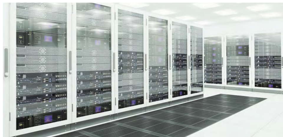
As its name implies, a Server Room is a space dedicated to the proper operation of a district’s servers. Environmental controls and security protocols are especially important for these spaces.
