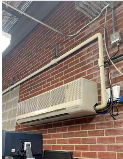
TRs require a dedicated Air Conditioning unit with independent controls. The split unit shown here works well for the space.
