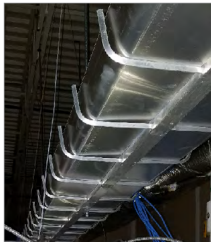
Closed metallic pathways used in exposed visible areas of egress.
