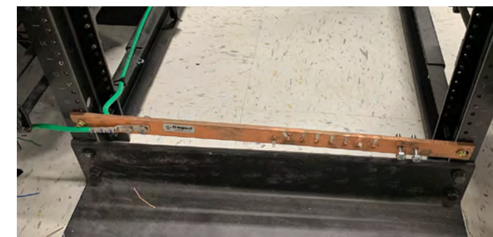
A Telecommunications Grounding Busbar (TGB) installed in an equipment rack as per industry standards.
