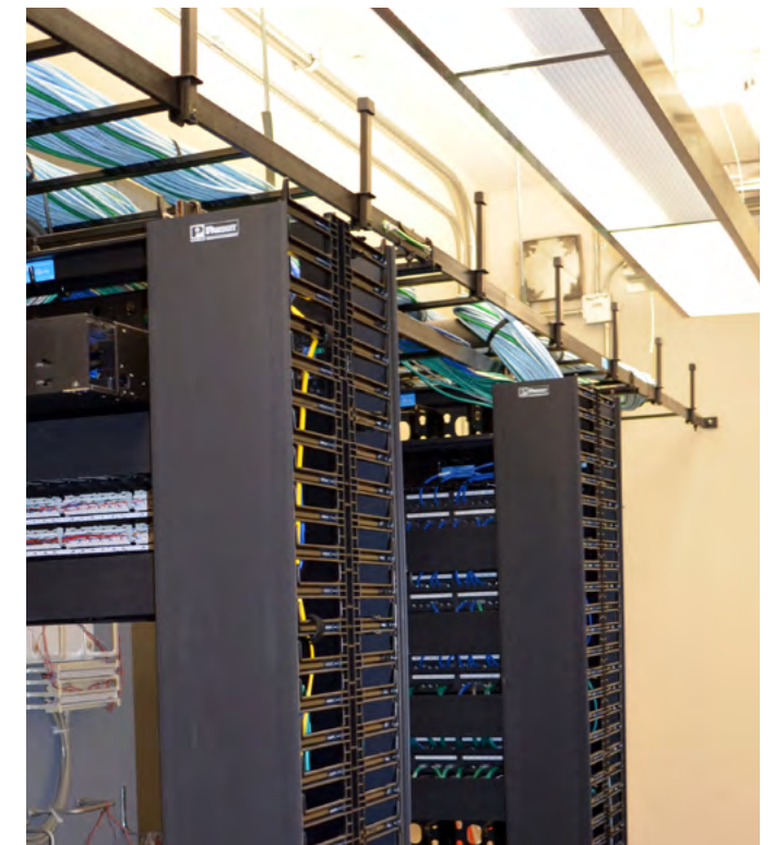
This TR has proper illumination as well as standards-compliant cable management, both overhead and at the racks.
