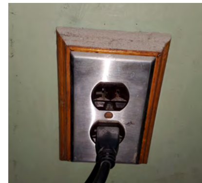
This outlet is not dedicated and lacks both emergency power and proper labeling.
