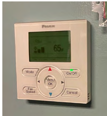
A standards-compliant, wall-mounted independent AC control unit in a TR.
