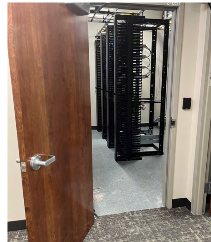
Entrance doors should swing out and have both card access and video surveillance.
