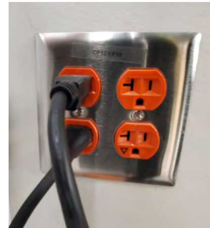
A dedicated electrical circuit with (2) 20A outlets (left) and an emergency generator outlet with proper labeling.
