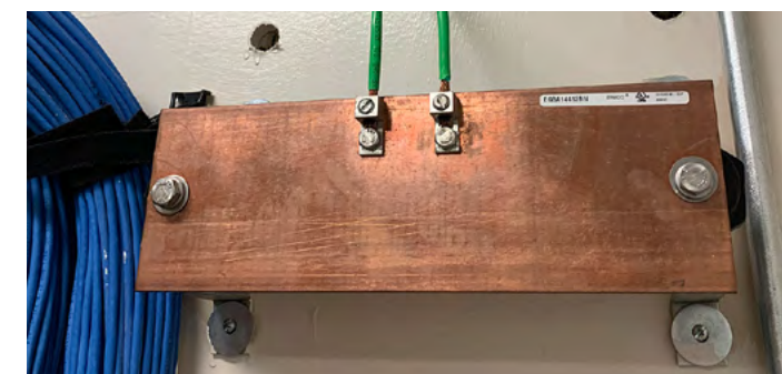
This Grounding infrastructure does not meet industry standards due to a number of deficiencies: undersized conductors, single-hole lug nuts, and no labeling.
