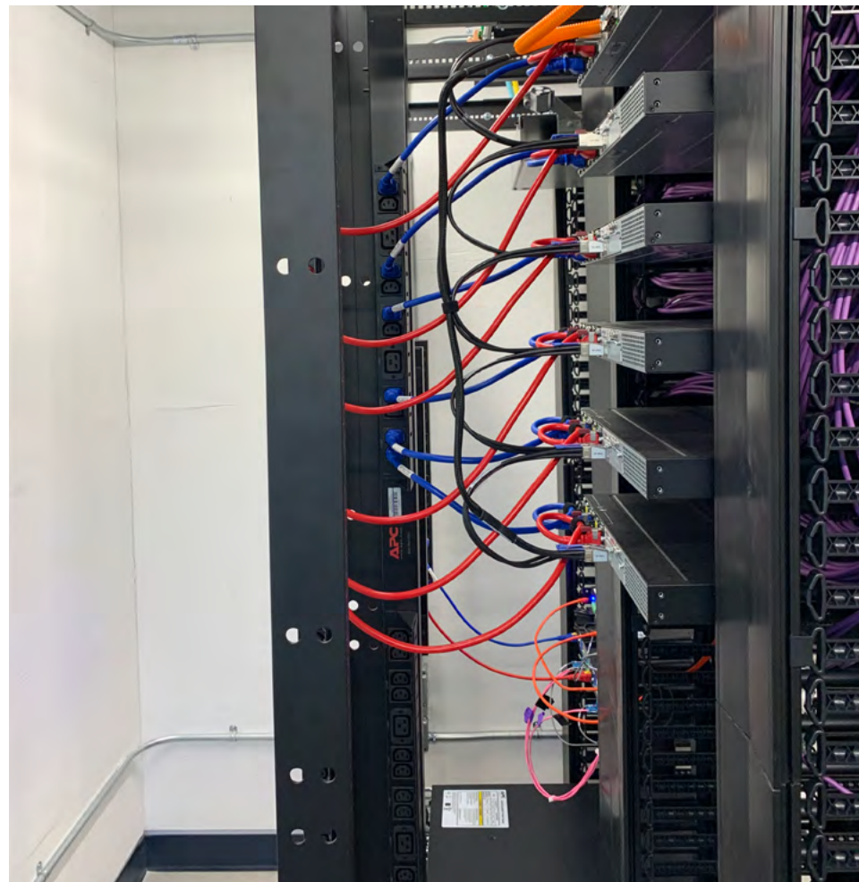
This TR meets all construction criteria including light color (linen) walls, adequate rack clearances, VCT flooring, and rack cable management.
