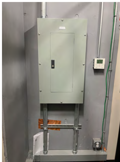
A dedicated electrical breaker panel should be installed in each TR.
