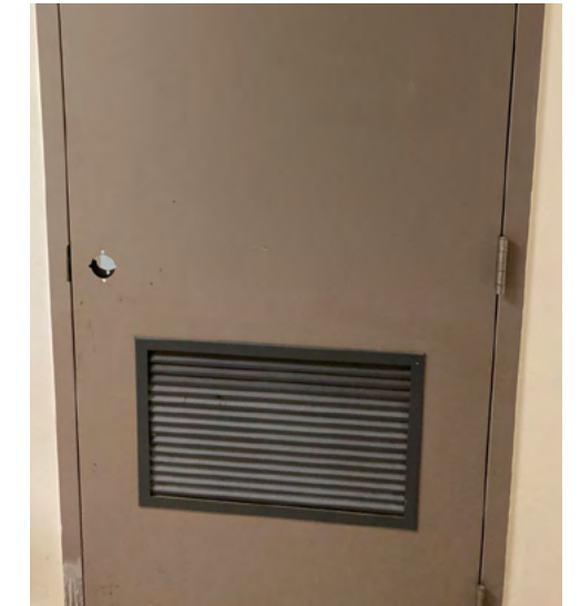
This TR exterior door lacks both a door knob and a locking mechanism.
