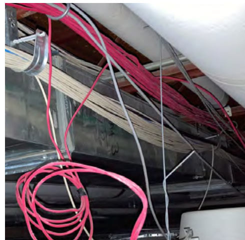
J hooks be spaced 4' apart and staggered 2 - 3" off center for each hook.
