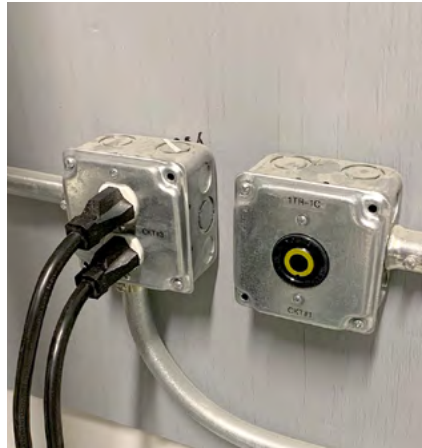
A dedicated electrical circuit with (2) 20A outlets (left) and a higher amperage twist-lock usually used for powering UPSs.
