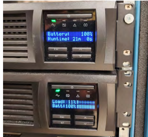
These two standards-compliant rack-mounted UPS units display adequate battery life and run times.
