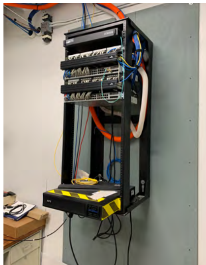
In this TR, the wall-mount open rack is mounted on properly treated, standards-compliant plywood.
